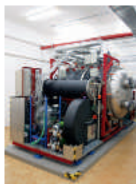
Picture 22: The multifunctional vacuum chamber (view from the opposite side).
