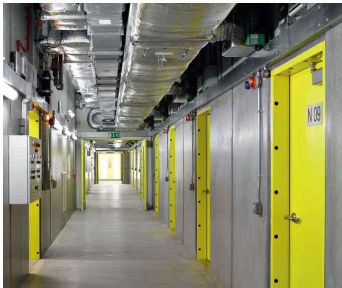
5. Corridor with nitrate cells to right and acetate to left in new MFS. ©BFI Photograph by Edmund Sumner
