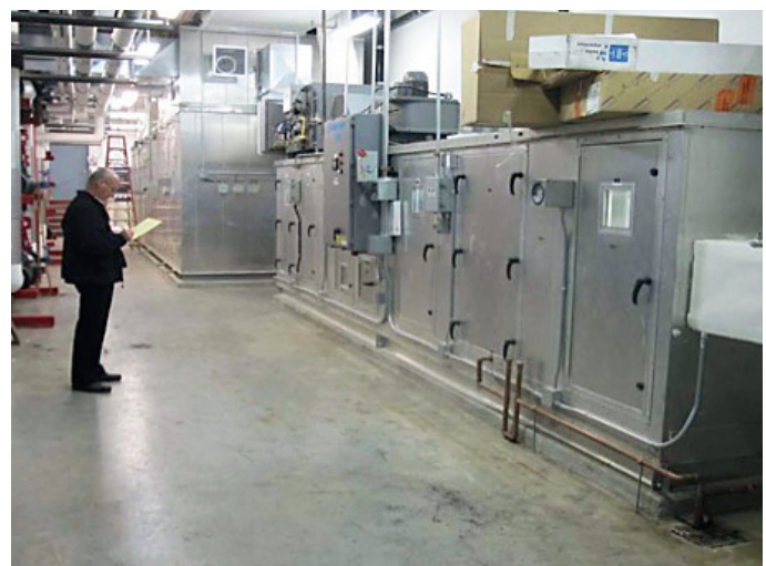
3. One of the AHUs at the Library Annex at Cornell University. Project partner Peter Herzog of Herzog/Wheeler & Associates is shown.
